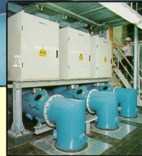
Voltage-transformer and capacitor cubicle
